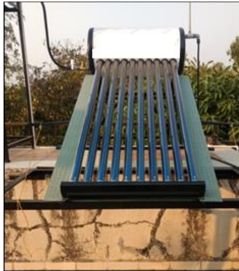
Fig. 1 Existing domestic solar water heater system
