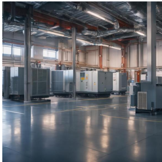
Fig. 2. Building with installed HVAC
