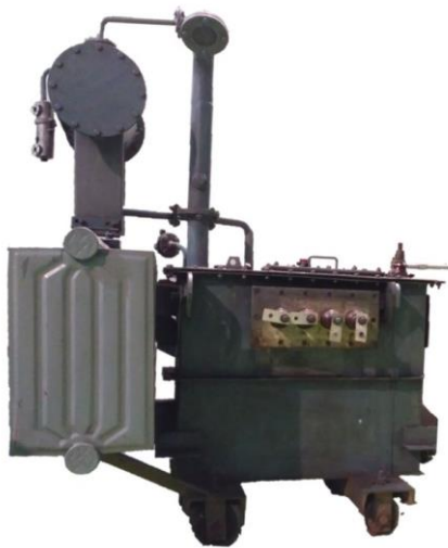
Fig. 3. 250kVA, 50Hz, 11kV delta-star connected distribution transformer
