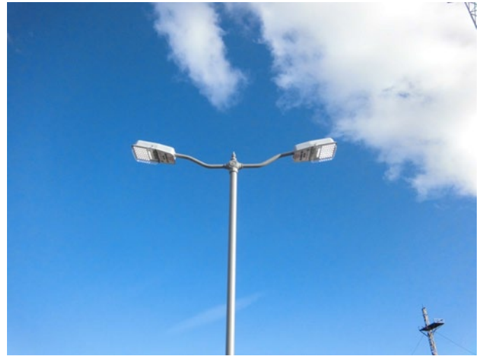
Figure 4. The streetlights used as a load
