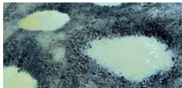
Fig. 1. Road surface: visual illustration of potholes
