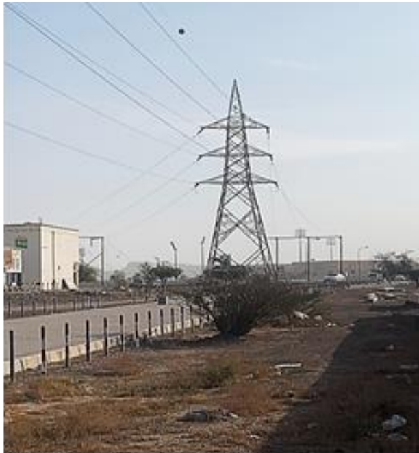
Figure 6. 132 kV Single conductor double circuit of Line 1
